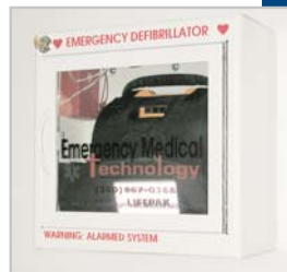
Eight AEDs have been installed in WCH work areas
